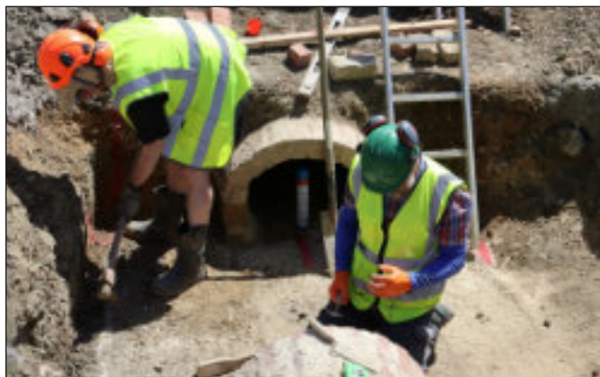
Dealing with the collapsed section of the bywash culvert
