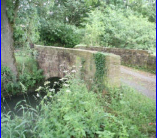
Silted up: the feeder from the Dane to Rudyard Reservoir
