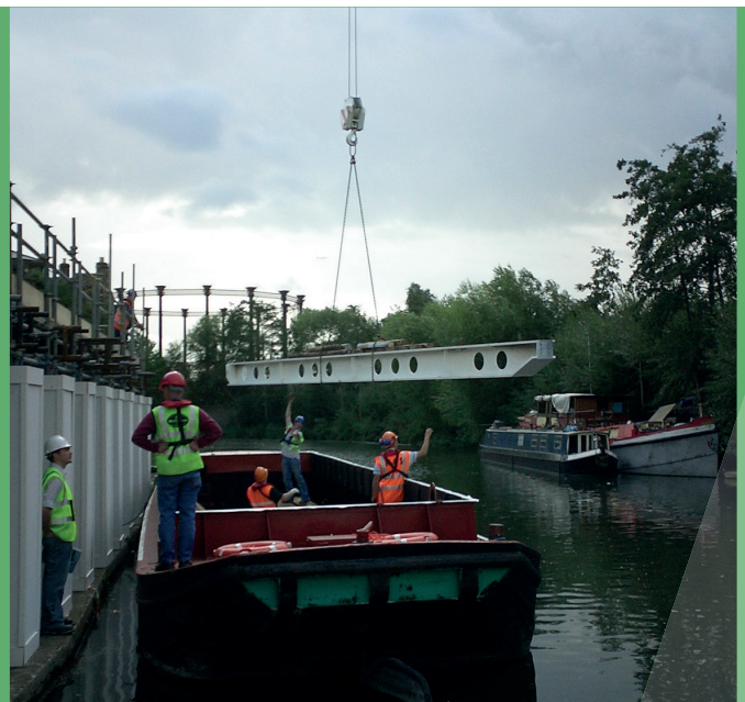
Wood Hall & Heward (WHH) Ltd delivering materials for the Kings Cross development in London for McAlpine.
