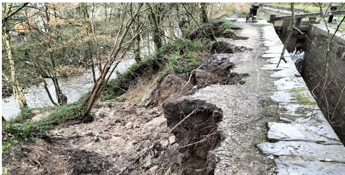
Embankment collapse at Lock 11 West, Huddersfield Narrow Canal (credit: Duncan Roberts)
