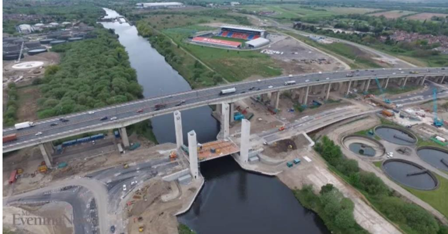
Manchester Evening News photograph of Salford Gateway Bridge after replacement of the fallen deck.
