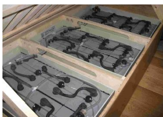
A Lead-Acid Traction Cell Installation
