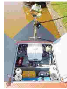
A Typical Generator Installation
