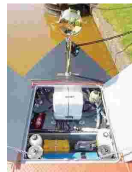
A Typical Generator Installation
