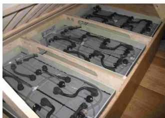
A Lead-Acid Traction Cell Installation
