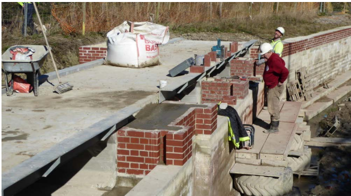
A make-shift work platform supported on old tyres, unstable, no edge protection or means of access.
