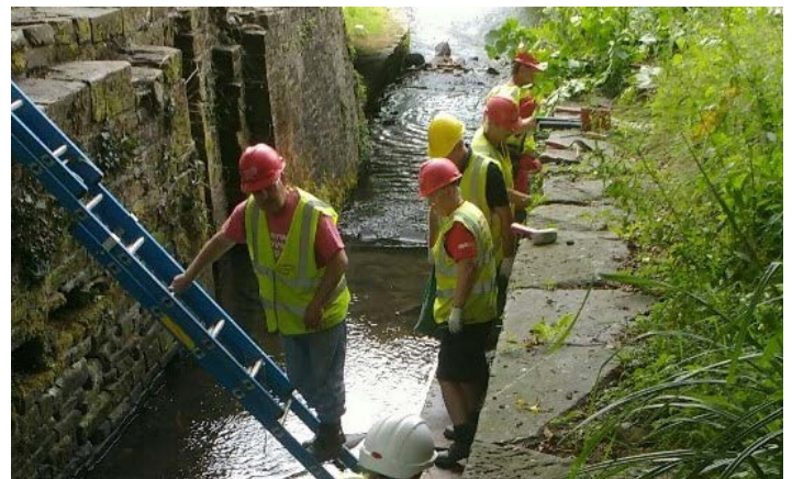
Working in a lock chamber on a platform with inadequate access or edge protection.
