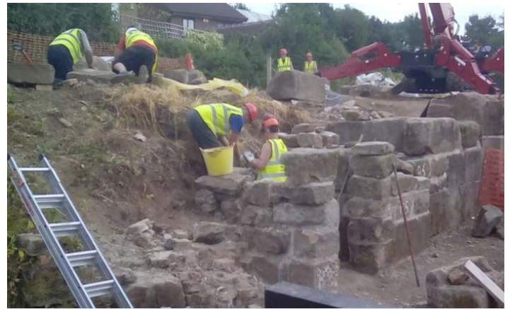
A partly restored lock with openings and unprotected edges.
