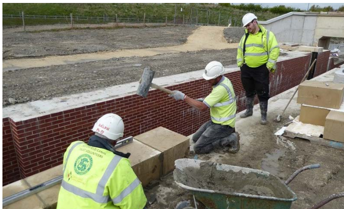
Installing copings to a finished lock chamber, no edge protection.
