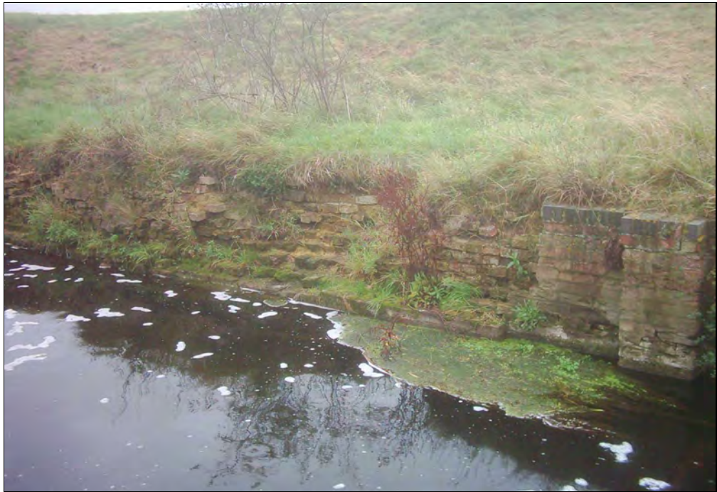
Photograph 10.1: Erosion of Tumby Lock Wall on East Side
