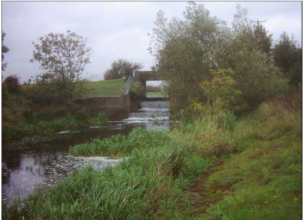
Photograph 10.2: Fulsby Lock's Present Condition
