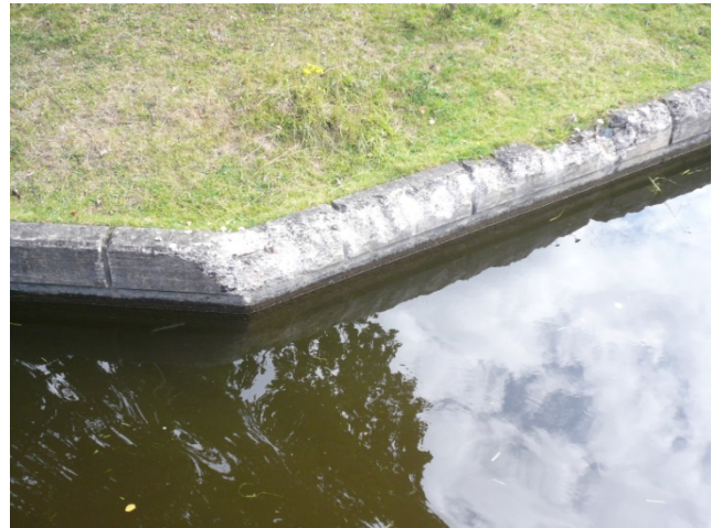
Note damage to edge – imagine damage to boats!
