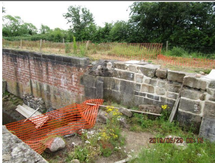
Anchor block in need of repair.
